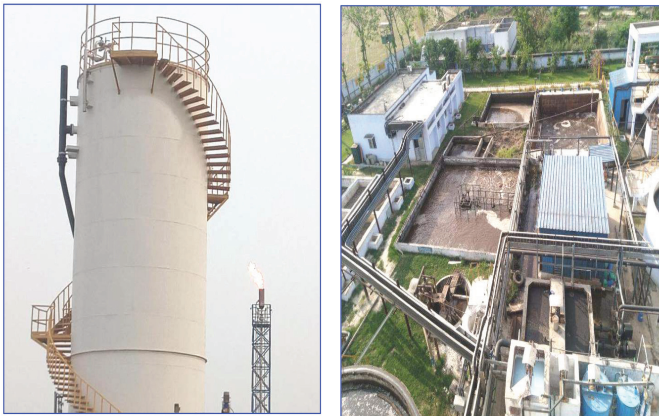
Figure 2 : Anaerobic reactor and ETP aerial view
