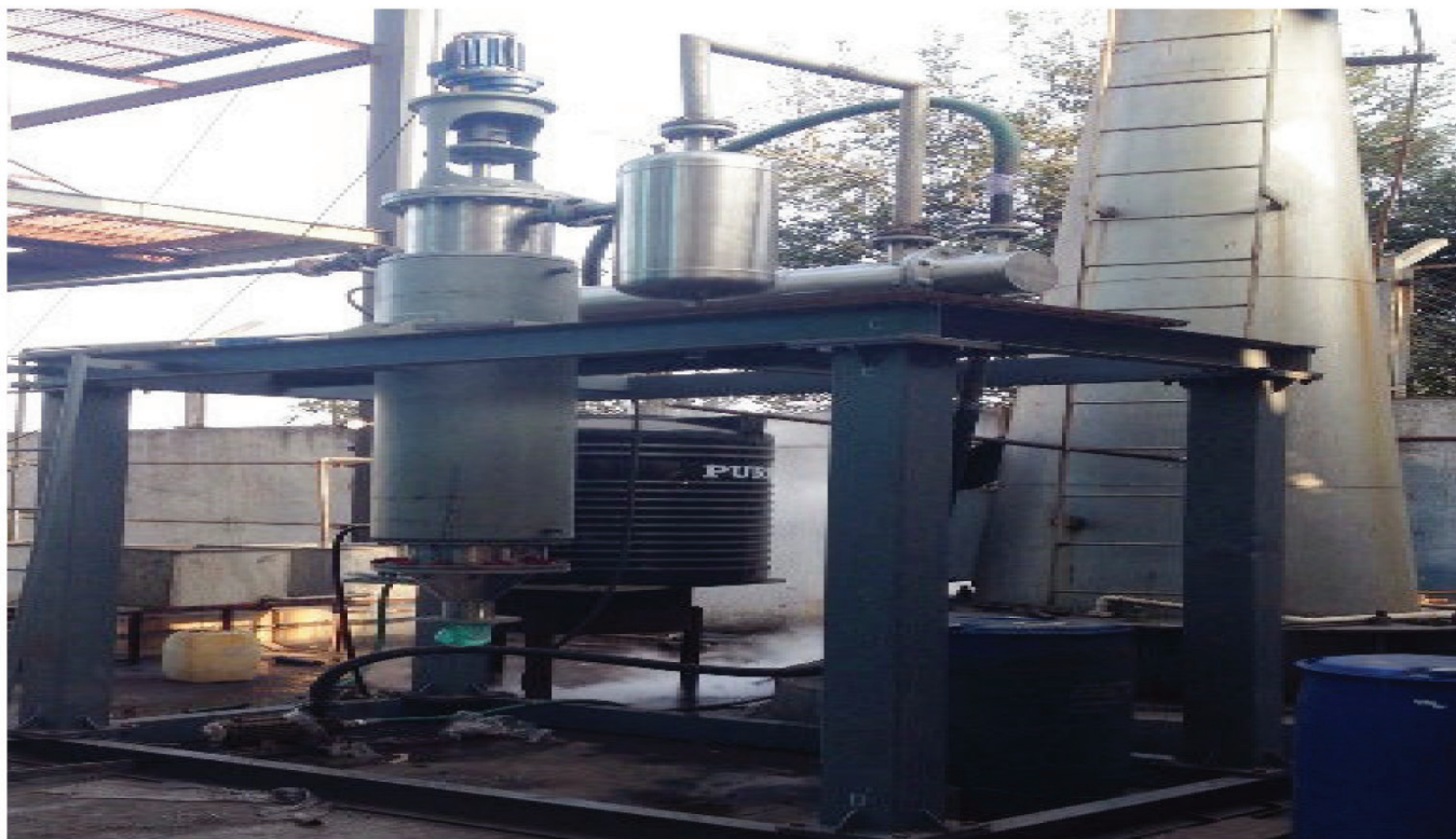
Figure 11 : ATFD Installation at SSM
