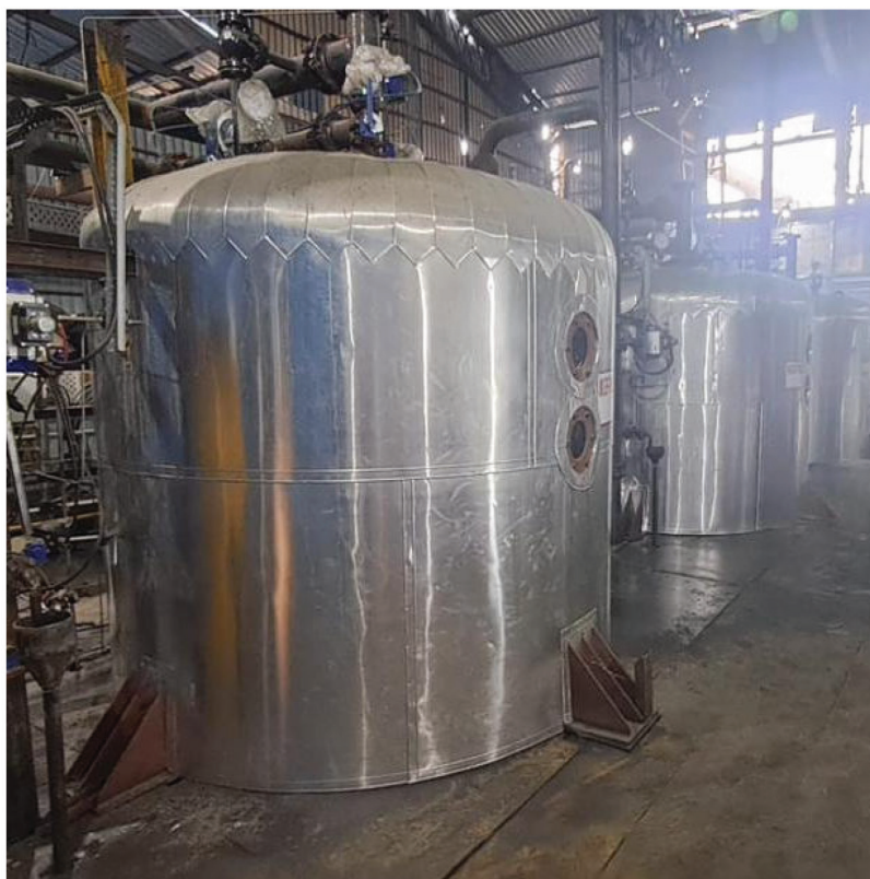
Figure 5 : Multi bed filtration system
